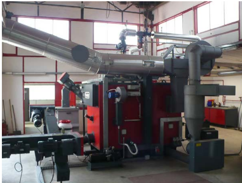
Modern, fully automated 500kW wood-fired boiler providing space heating for a factory, Bärnbach, Austria
