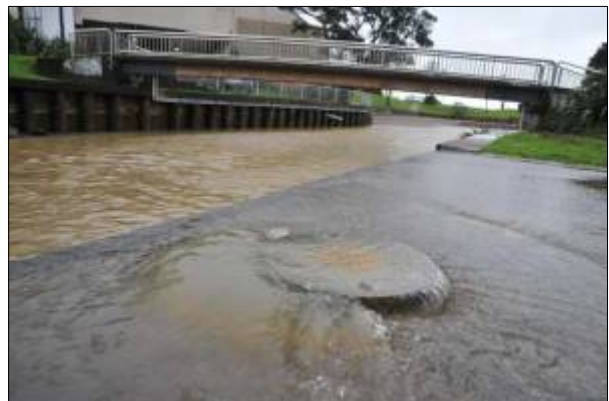
Figure 12: Wet weather overflow in Browns Bay in July 2008
