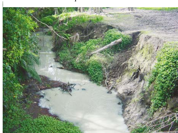
Figure 3: Lucas Creek eroding due to development pressures
