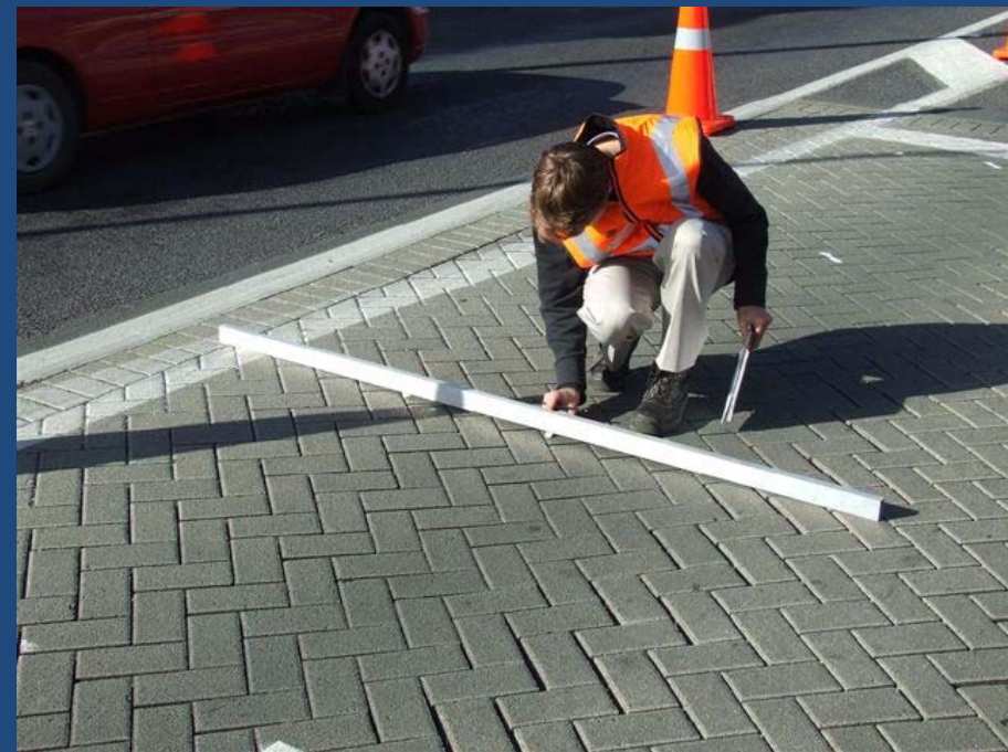
Figure 3: Pavement rutting measured with a 2-m straight edge
