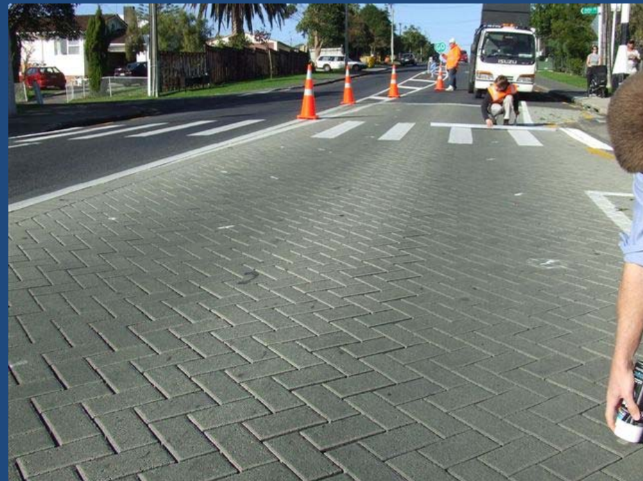
Figure 4: Rut measurements taken at 2-m intervals along the pavement
