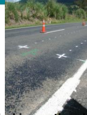
Flushing on the wheel paths of a pavement
